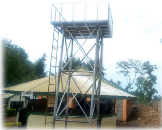
Figure 3: Erected water tower to hold 5000 litres tanks to supply maternity and ANC units.
