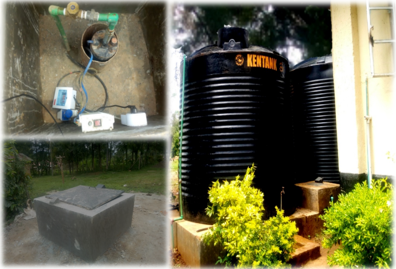
Figure 2: Complete sealed borehole connected to the solar powered pump (L), water connection to the 10,00 litres tank (R).
