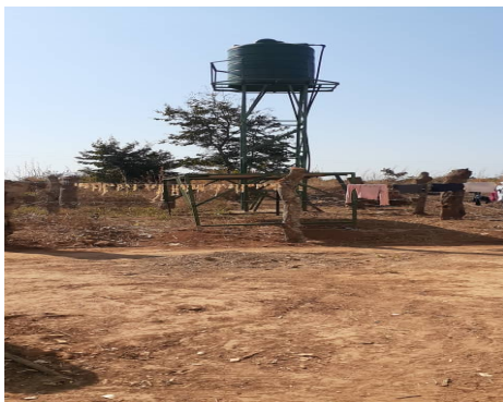
Solar powered borehole
